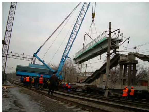
Unloading of spans from railway platform and assembly of the spans on the site.
