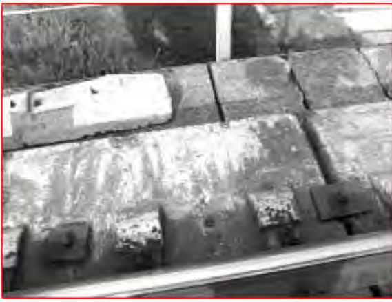
Slackening of tension or breaking of pins and as a result, damage of joints.
