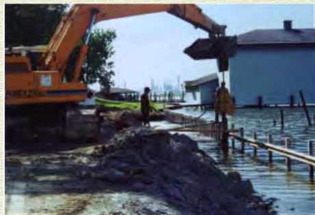
Step 7: Profiles' installation on the site to the bearing composite basic structure
