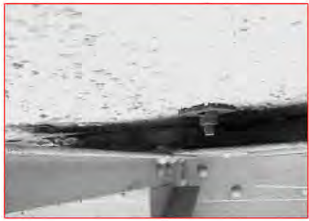
Spalling and destruction of the reinforced cement-sand layer Rot damage and destruction of a layer of plates.
