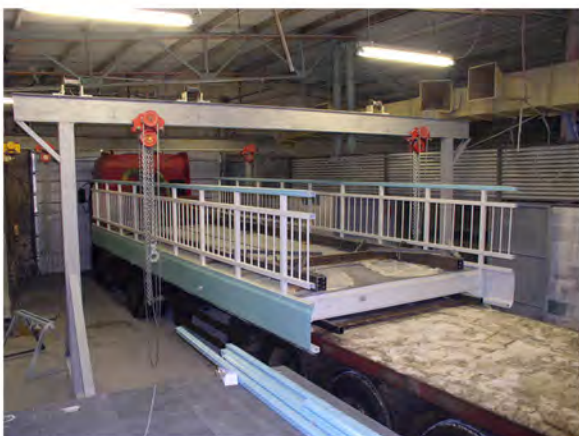
Loading of the finished bridge span at the warehouse of the enterprise
